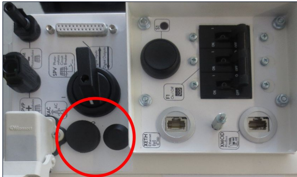
Illustration 15: Blanking plugs on the storage system
